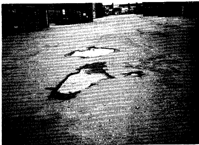
Damage from heavy container handling equipment
