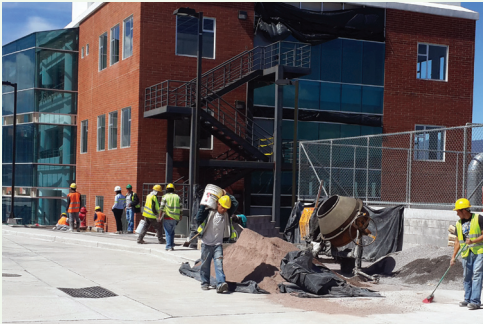
UNOPS construction at the IGSS Regional Hospital of Quetzaltenango, Guatemala. Photo: ©UNOPS
