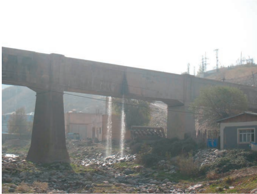
Photo 7.1: Damaged water bridge, Dushanbe
