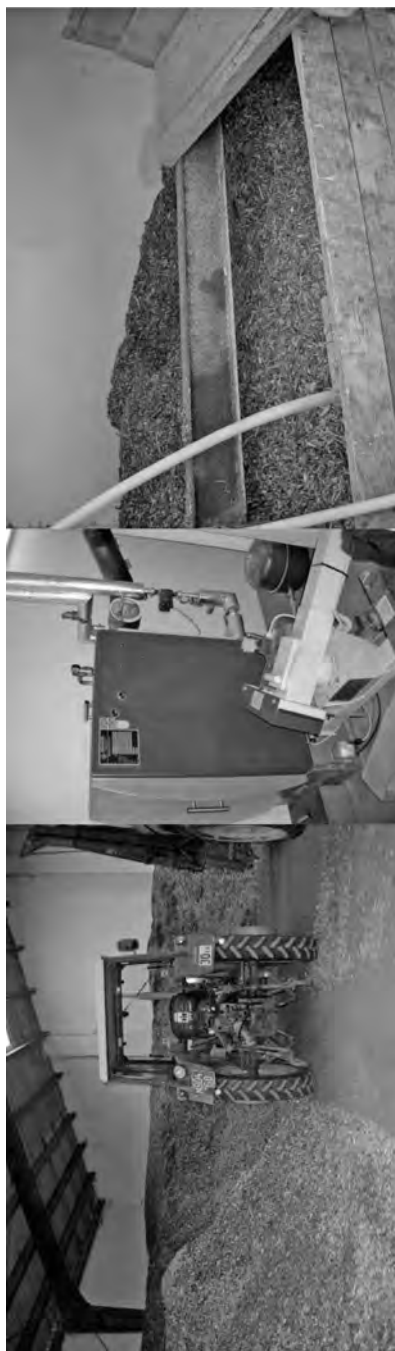
Plate 5.1.1 Photo of a former barn used as additional storage facility for wood chips (left). Photo of the biomass boiler (centre). Photo of the indoor woodchip storage beside the boiler (right). ( Source: © K. Aoki and F. Kraxner)
