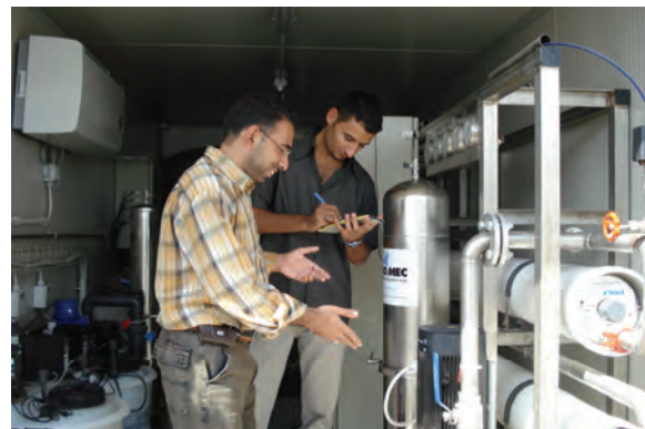
Figure 5 Water treatment equipment installations
