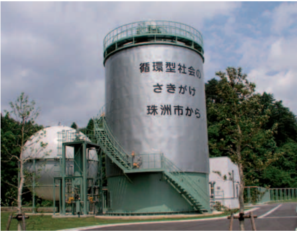
Photo 1. Methane fermentation tank
