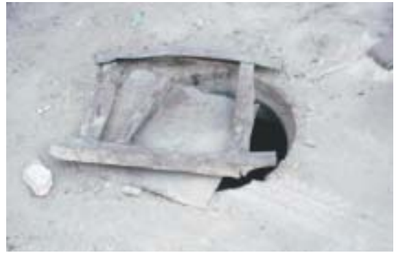
Manhole damaged by tank in the centre of Jenin
