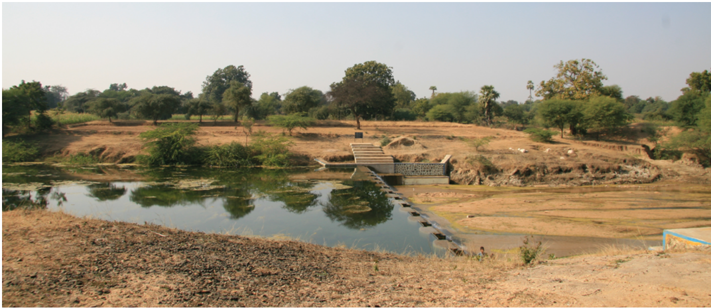
An eco-friendly check dam is used to harvest rainwater for irrigation in Rajasthan, India. © Govindasamy Agoramoorthy / Shutterstock
