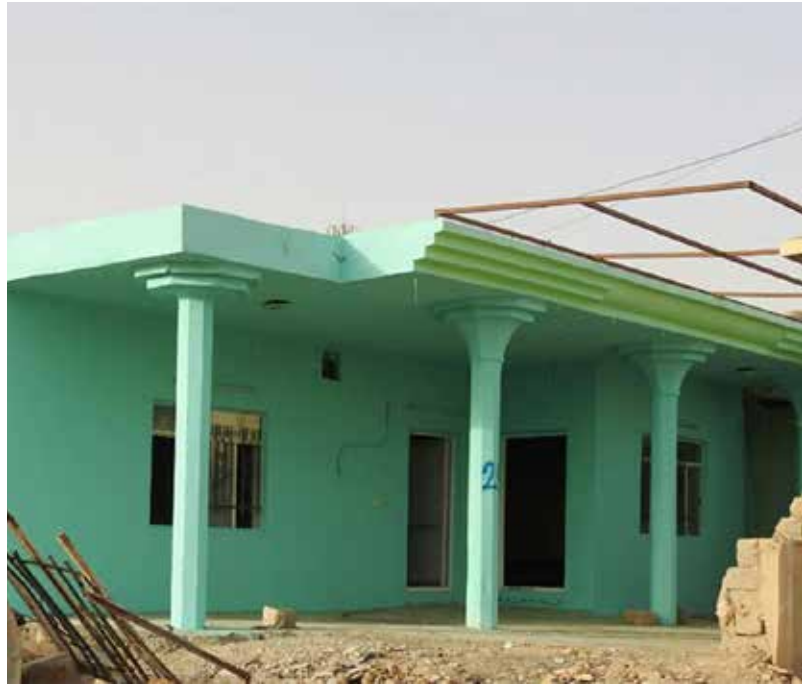
Top Left Image: Before (damaged house). Top Right Image: After (Rehabilitated house).
