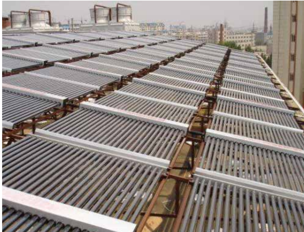
Image: Industrial system solar water heater. © UN-Habitat
