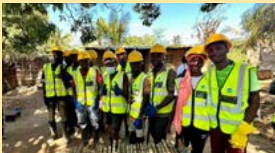
Pemba, Mozambique: A group of young people wear hard hats and yellow vests, they are displaced people and longtime residents of Alto Gingone. A partnership with WFP and AVSI has enabled them to work together, learning to improve the drainage system in their neighborhood. UNRCO/Helvisney Cardoso
