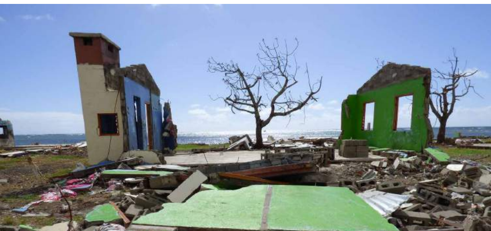
Damage caused by Category 5 Cyclone Winston in Koro, Fiji. Even concrete and brick buildings had collapsed.
