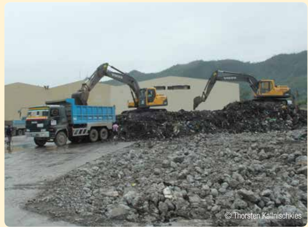
Temporary dumpsite, Tacloban Abucay
