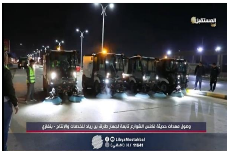
Figure 12.1 Road Maintenance in Benghazi
