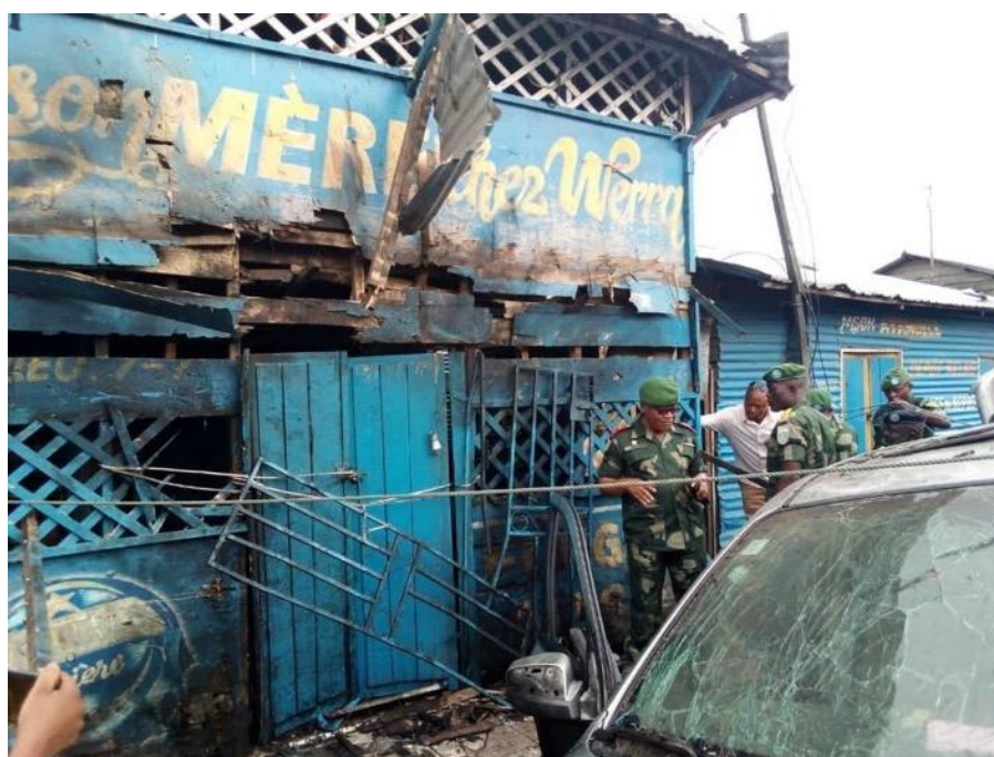
Picture of the bar where the explosion took place, provided by a FARDC source
