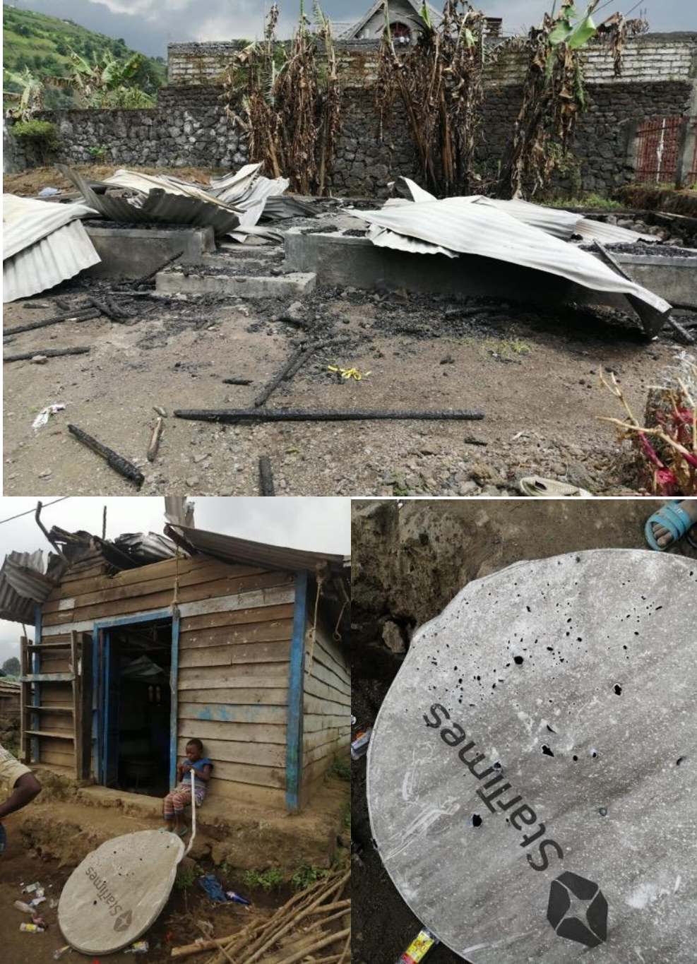
Pictures of houses and infrastructure impacted by the shelling, taken by the Group on 9 June 2022
