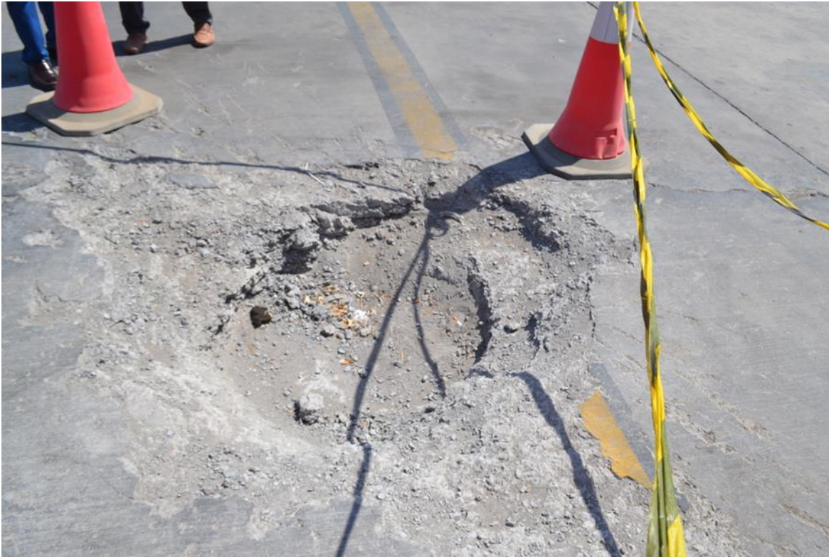
Figure 7.5 Impact point of the second missile on the runway
