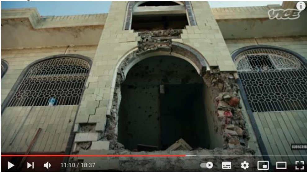
Figure 35.2 Damages to the Club
