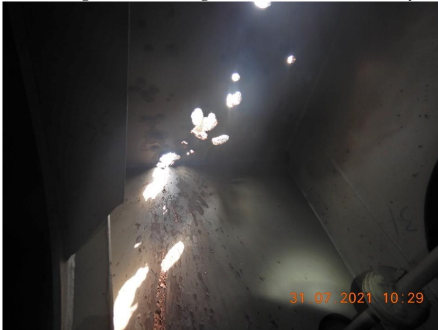
Possible fragmentation damage in the roof of the main cavity
