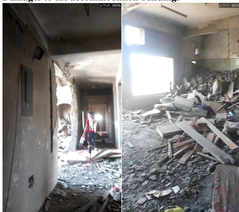
Figure 33.3 Damages to the accommodation buildings
