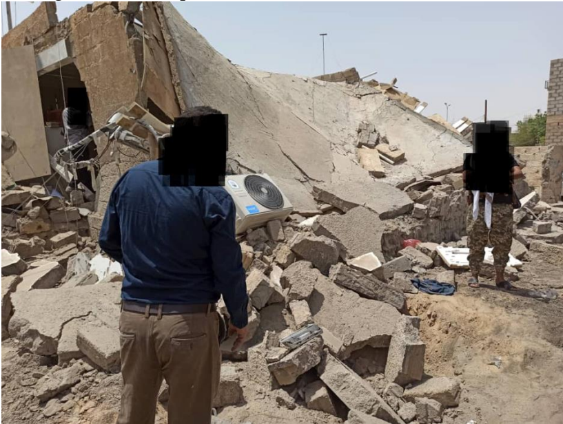
Figure 35.13 Damage to the Mosque
