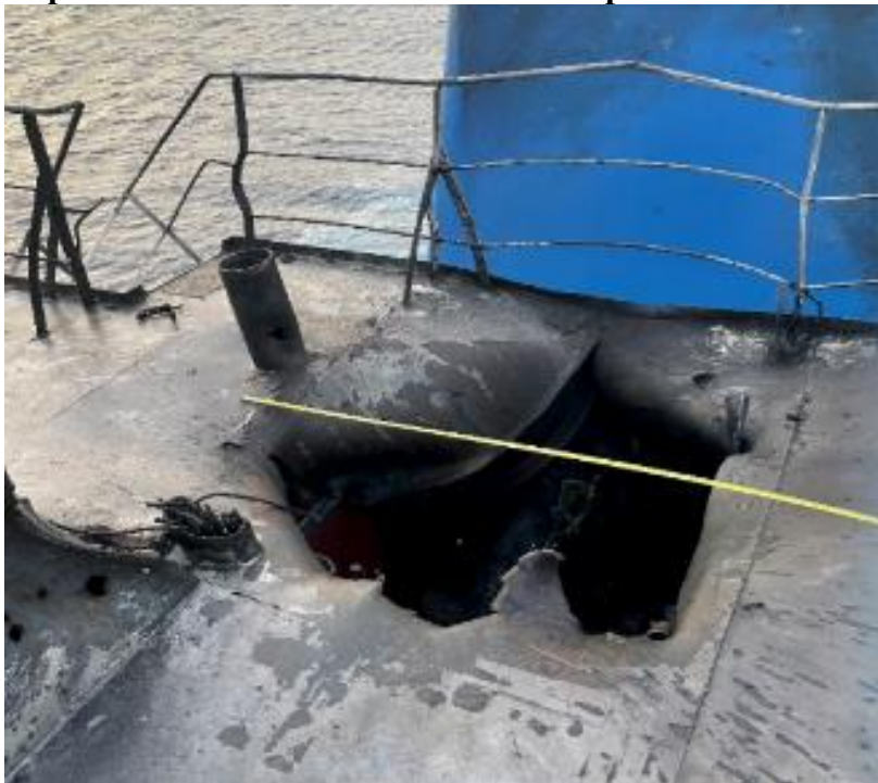
Figure 15.2 Impact location of the UAV on the aft superstructure
