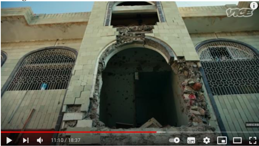
Figure 35.2 Damages to the Club
