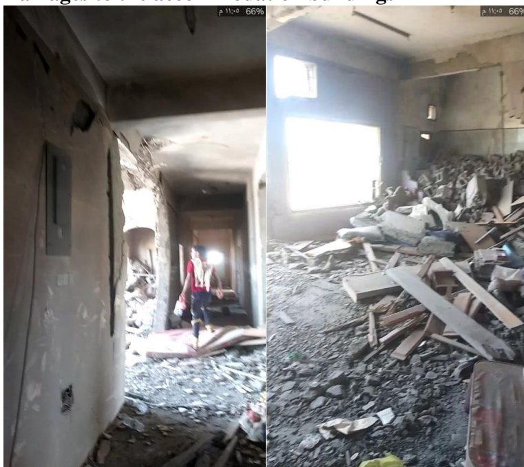
Figure 33.3 Damages to the accommodation buildings
