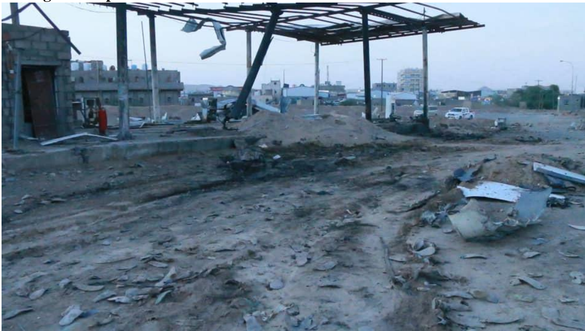
Figure 35.10 Damage to the petrol station
