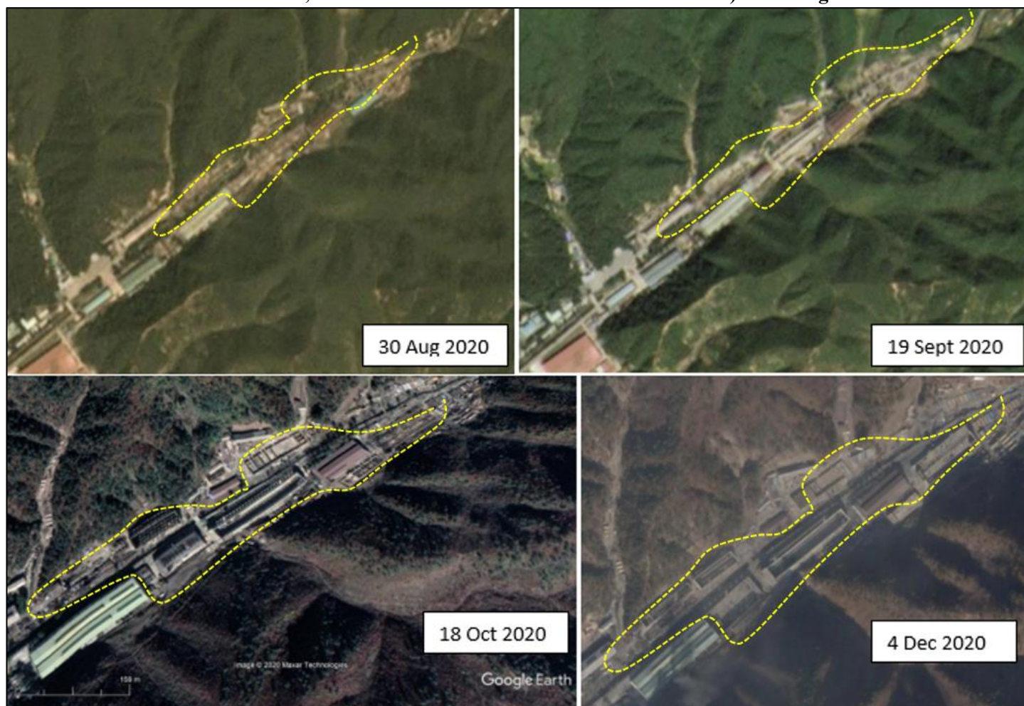
Figure 13-4: Demolition of several buildings and new construction on the site NE (southwest corner: 40^{\circ} 03' 47'' N 125^{\circ} 13' 47'' ; northeast corner: 40^{\circ} 03' 56'' N 125^{\circ} 14' 08'' E) from Aug 2020
