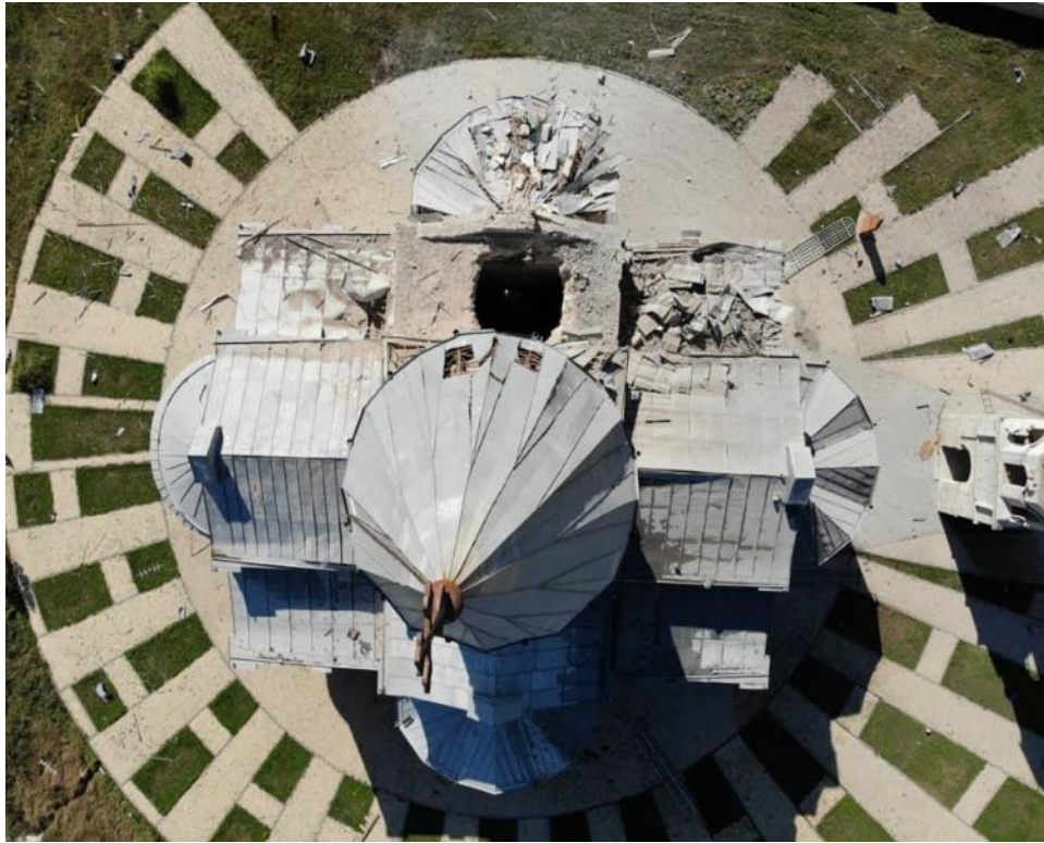
Images 1-4: The damage caused to the Holy Savior Ghazanchetsots Cathedral following the two strikes on 8 October 2020
