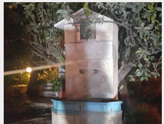
Public water standpipe in a Beirut suburb.
