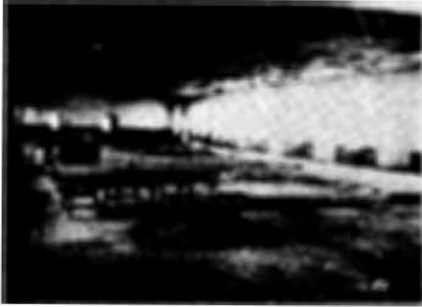
Nos. 25 and 26. Shows the interior of two well-built buildings, which was probably intended for packing or other light manufacturing work. It has been very badly stripped. The window frames were all torn; holes were made in the ceiling.
