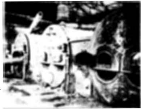
Nos. 32, 33 and 34 are the new boilers installed in the boiler unit. These boilers are new and some of them are equipped with automatic stokers.
