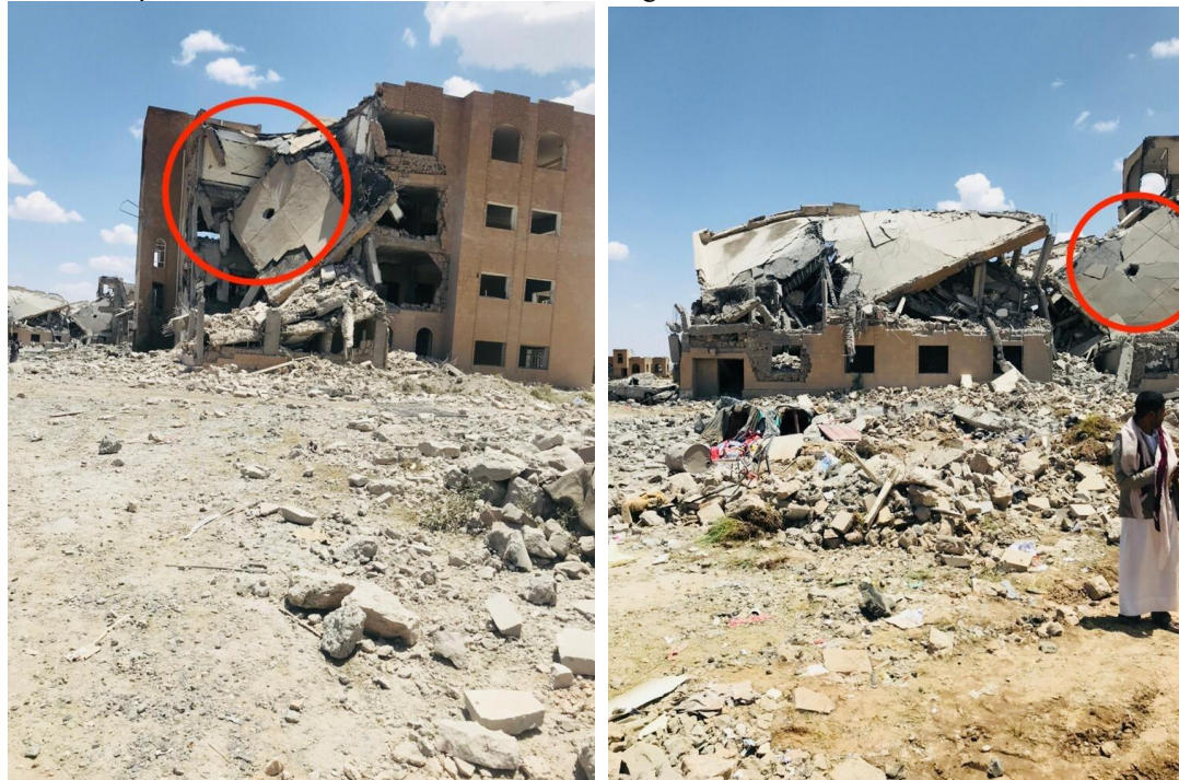
Figure 3 Point of impact of aerial bomb in two different buildings
