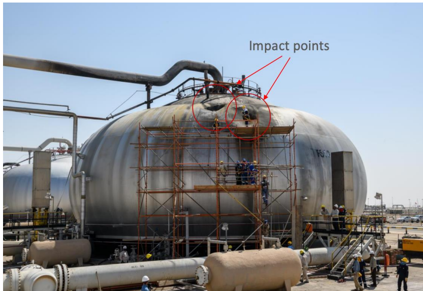
Figure 14.1 Damaged separator tank in Abqaiq
