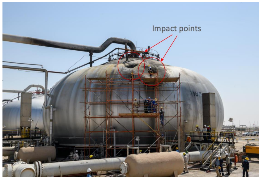
Figure 14.1 Damaged separator tank in Abqaiq
