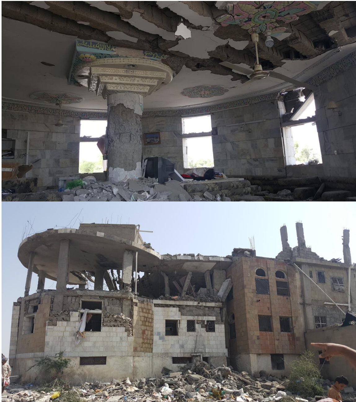
Figure 2 House after the incident
