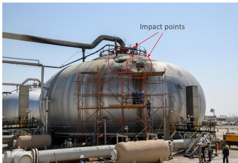
Figure 14.1 Damaged separator tank in Abqaiq
