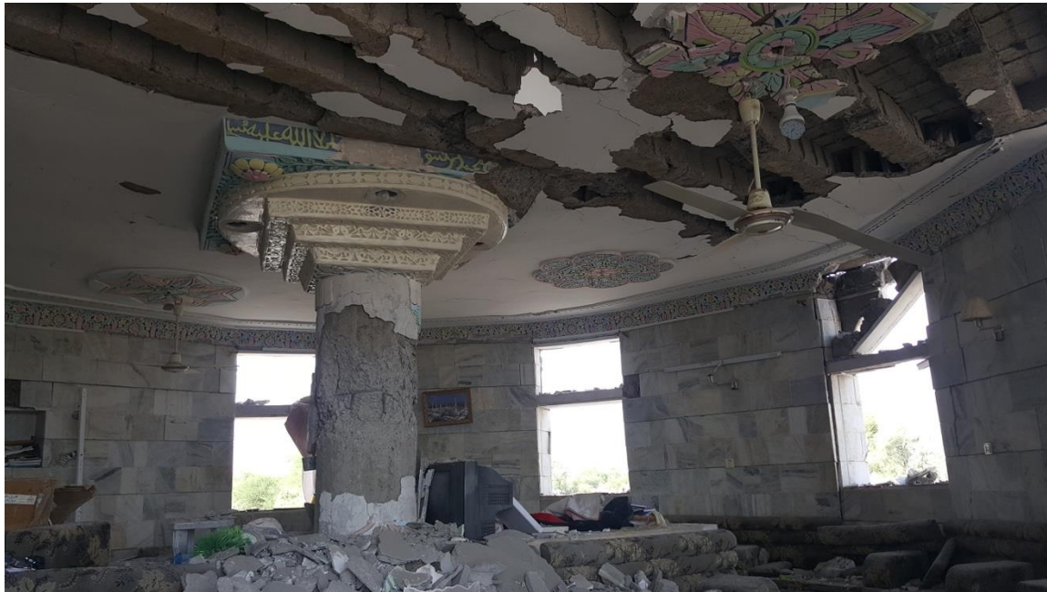
Figure 2 House after the incident
