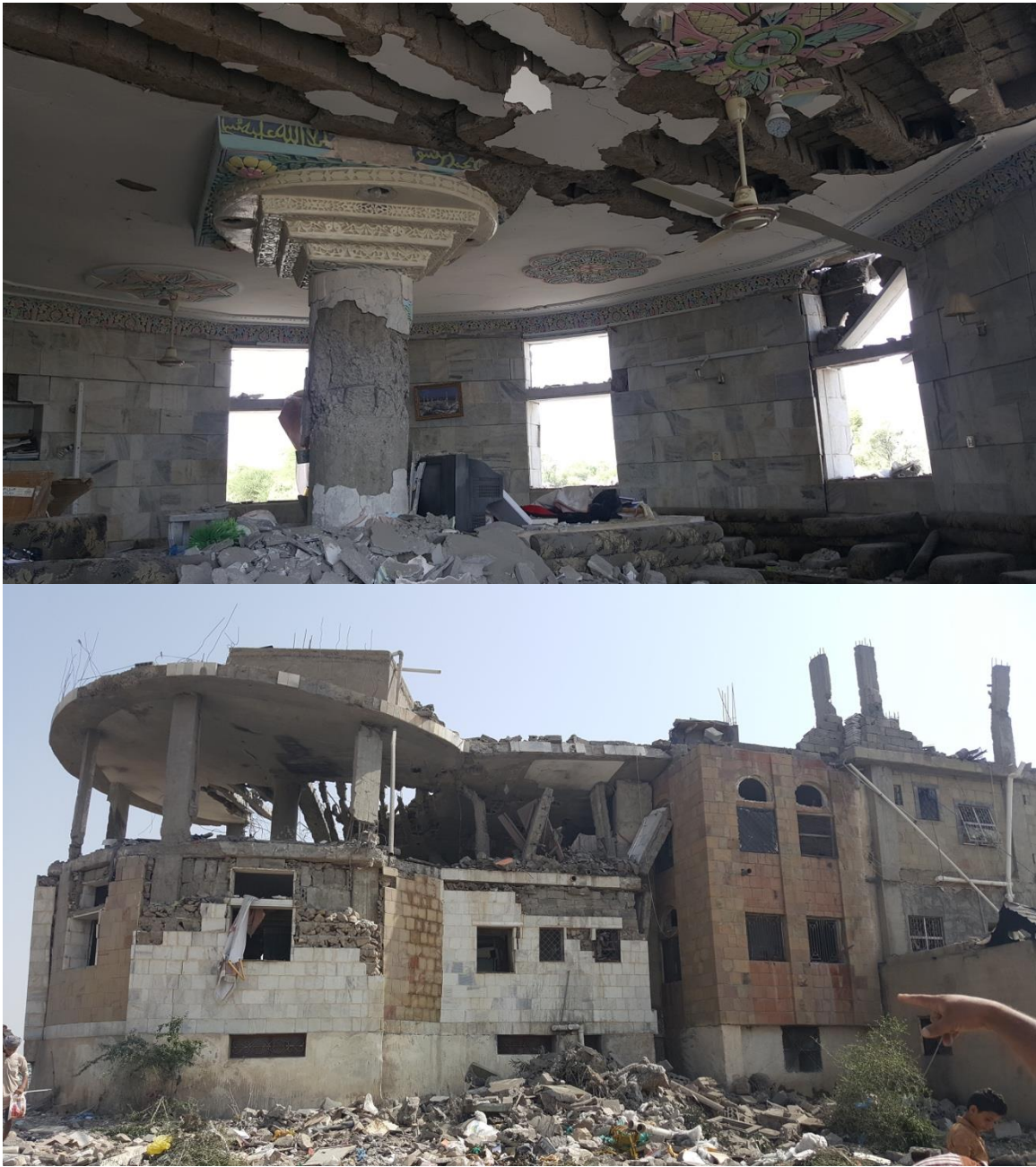
Figure 2 House after the incident
