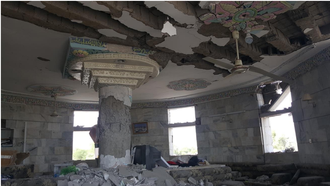
Figure 2 House after the incident
