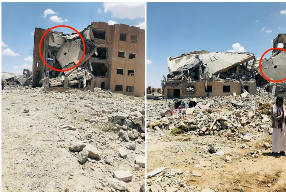
Figure XII Point of impact of aerial bombs in two different buildings of the Dhamar community college compound
