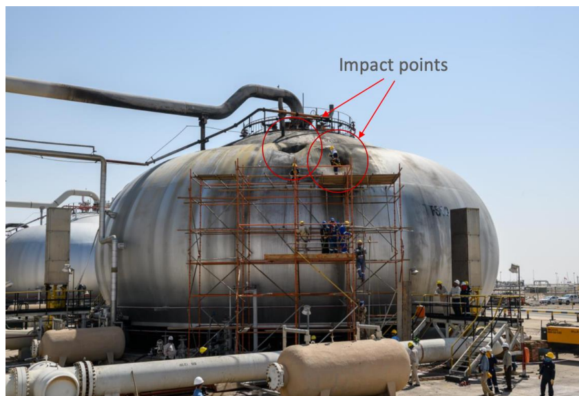
Figure 14.1 Damaged separator tank in Abqaiq
