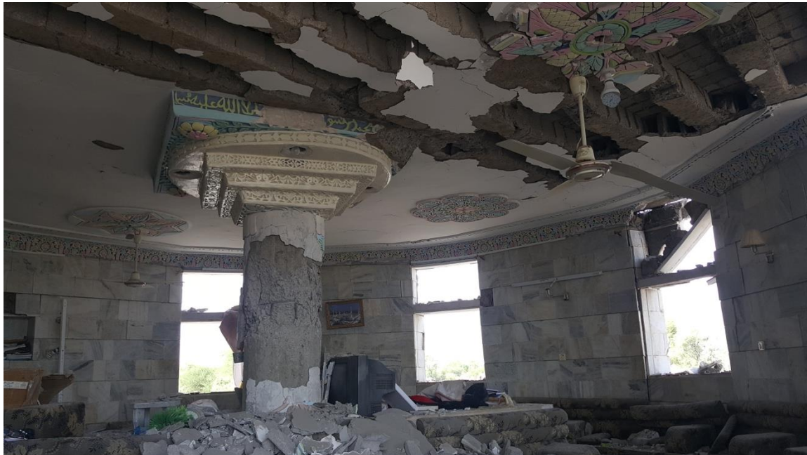
Figure 2 House after the incident
