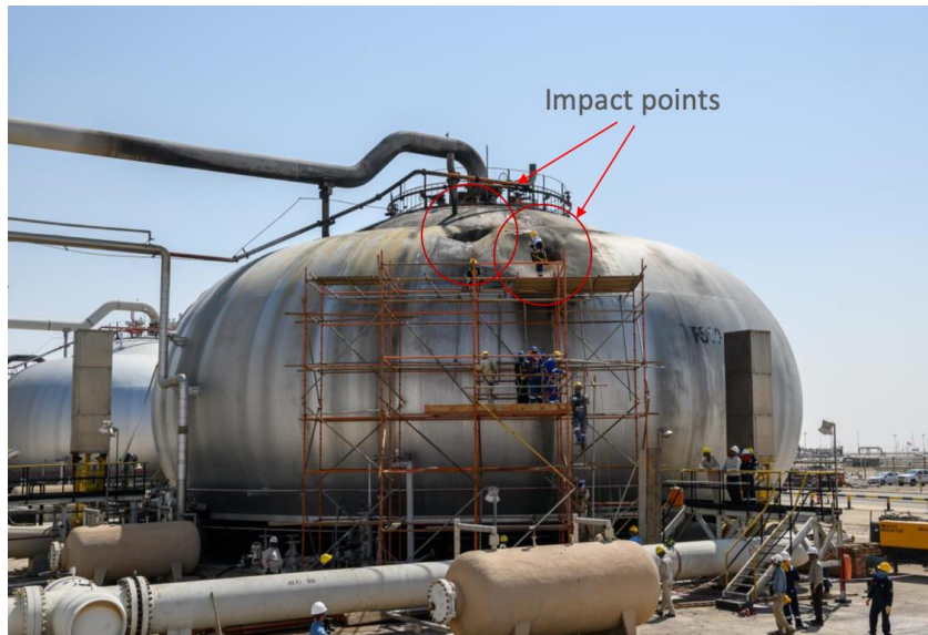
Figure 14.1 Damaged separator tank in Abqaiq
