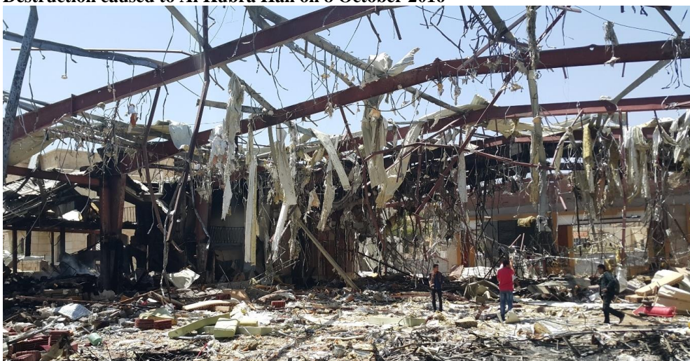
Figure II Destruction caused to Al Kubra Hall on 8 October 2016 2
