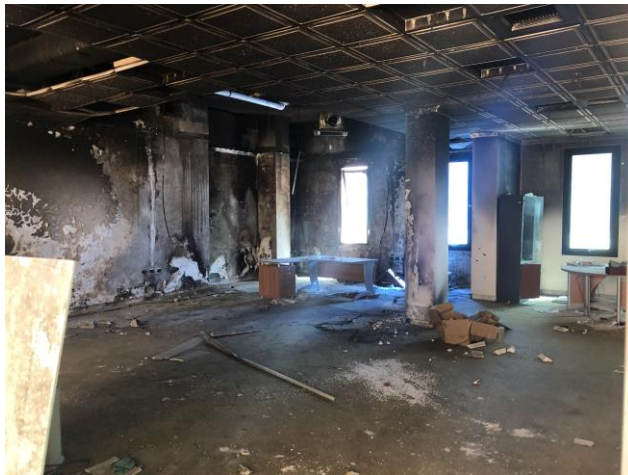
Figure 9.3 Condition of the premises in September 2019
