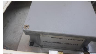
Image 51.22 ATS Servo Control Unit
