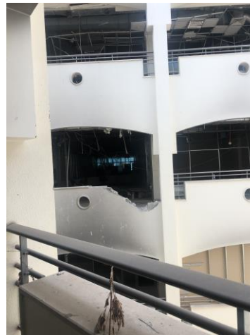
Figure 9.4 Condition of the premises in September 2019
