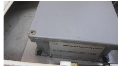
Image 51.22 ATS Servo Control Unit
