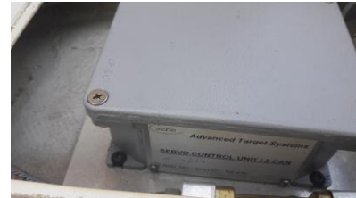
Image 51.22 ATS Servo Control Unit
