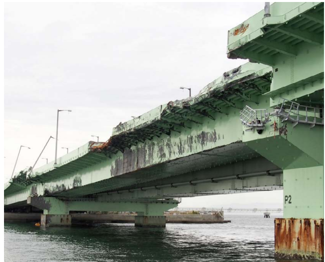
FIGURE 3: Damaged Access Bridge caused by Typhoon Jebi – Kansai International Airport
