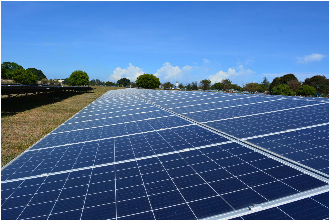
FIGURE 3: Solar PV system at Moi International Airport. Mombasa, Kenya
