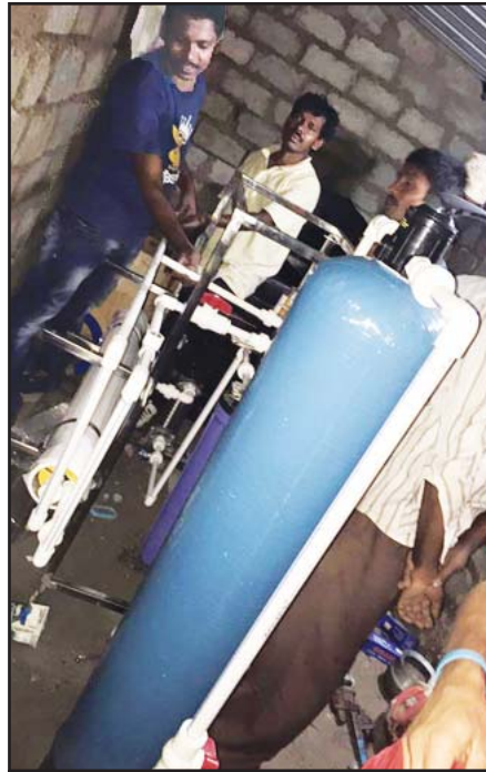
Community water filtration plant
