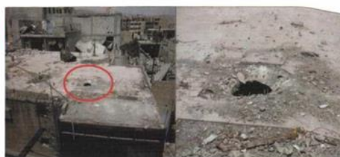
Presence of more than one crater of very similar appearance in concrete slabs on top of nearby buildings
