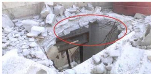
A crater in the roof has dimensions of 166 x 105 cm The presence of fragments of mild steel rebar inside the crater and wire netting indicates that it has been widened mechanically and intentionally
