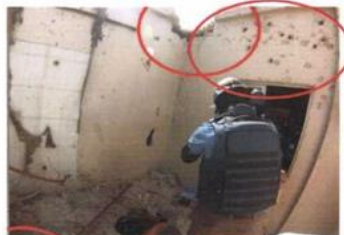
Traces of blast fragmentations on the balcony's walls
