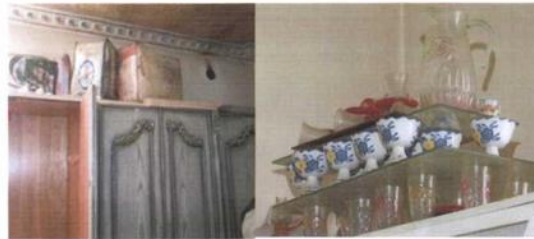
The penetration of the cylinder inside the top floor apartment does not allow its subsequent deflection laterally post-impact within the room without causing related damage to the furniture, floor, walls and windows of the room
