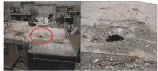
Presence of more than one crater of very similar appearance in concrete slabs on top of nearby buildings
