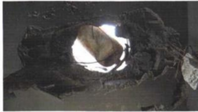
Black scorching on the crater and the destruction of steel rebar inside the aperture
