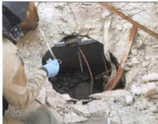
The shape and dimensions of the resulting aperture are consistent with the penetration of a solid body through the reinforced concrete barrier under the angle of 80-90 °
