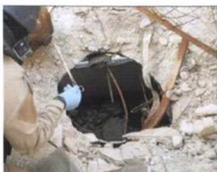
The shape and dimensions of the resulting aperture are consistent with the penetration of a solid body through the reinforced concrete barrier under the angle of 80-90 °
