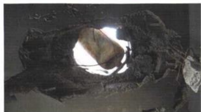
Black scorching on the crater and the destruction of steel rebar inside the aperture
