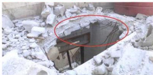
A crater in the roof has dimensions of 166 x 105 cm The presence of fragments of mild steel rebar inside the crater and wire netting indicates that it has been widened mechanically and intentionally
