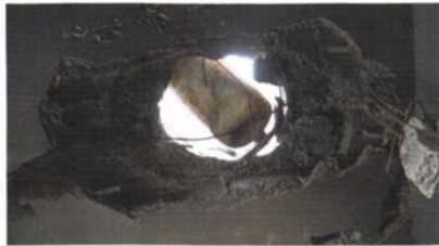
Black scorching on the crater and the destruction of steel rebar inside the aperture
