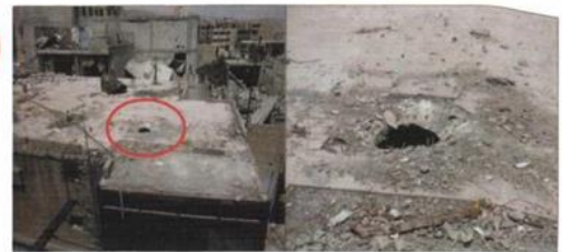
Presence of more than one crater of very similar appearance in concrete slabs on top of nearby buildings
