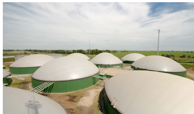
Source: Biogas plant, by buhanovskiy.
