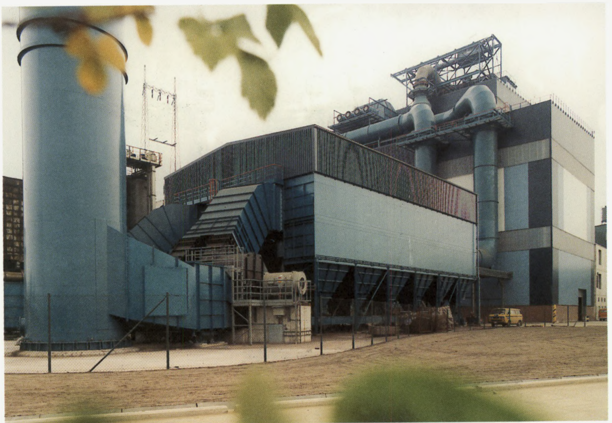
Photo 15: Bag filter dust collection at electric arc steel plant (producing stainless steel)
