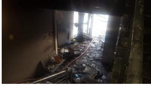
Figure 37.1 Damage to the hospital 149
