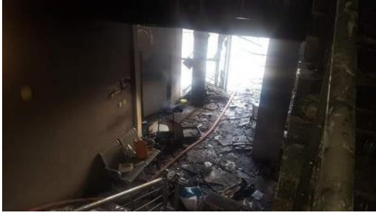
Figure 37.1 Damage to the hospital 149
