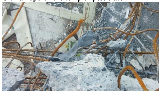
Figure D.60.5 Civilian apartment complex post blast
