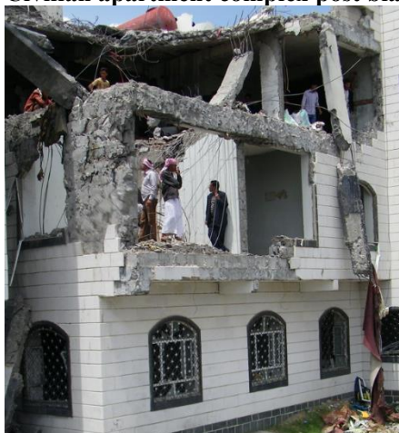
Figure D.60.4 Civilian apartment complex post blast
