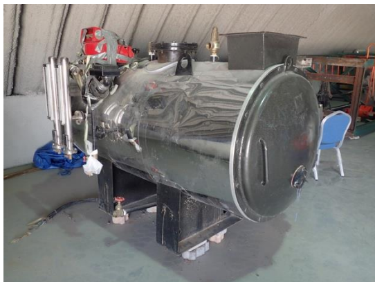
Figure D.36.7 Pressure vessel
