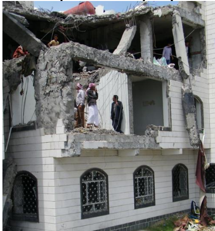
Figure D.60.4 Civilian apartment complex post blast
