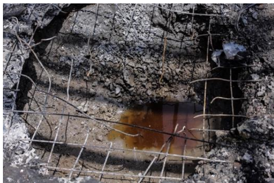
Figure A.60.5 Damage at impact point of EO 6
