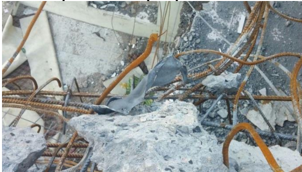
Figure D.60.5 Civilian apartment complex post blast
