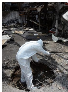
Figure A.60.6 Damage at impact point of EO
