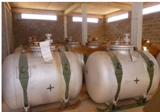
Figure D.36.11 Liquid bi-propellant oxidiser field storage tank 34
