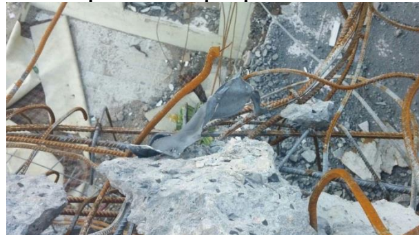
Figure D.60.5 Civilian apartment complex post blast
