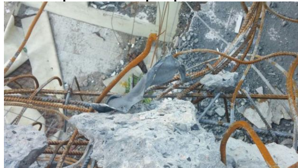
Figure D.60.5 Civilian apartment complex post blast
