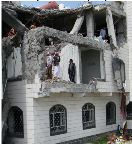
Figure D.60.4 Civilian apartment complex post blast
