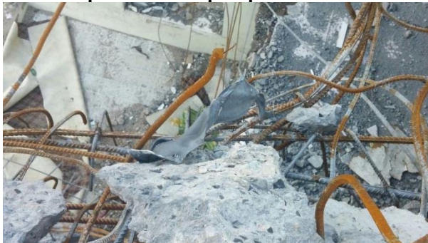
Figure D.60.5 Civilian apartment complex post blast
