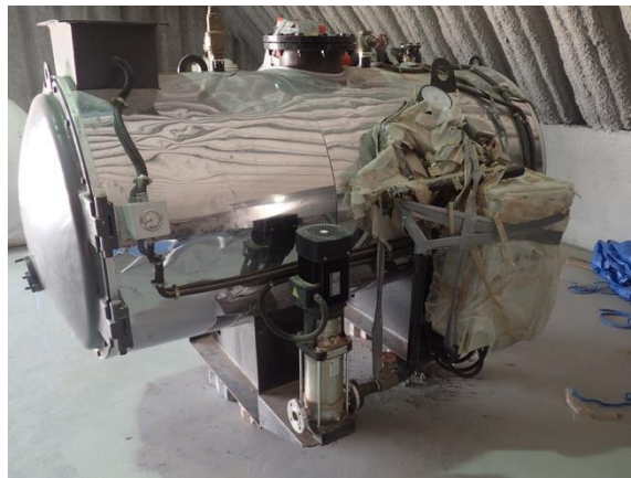
Figure D.36.6 Pressure vessel
