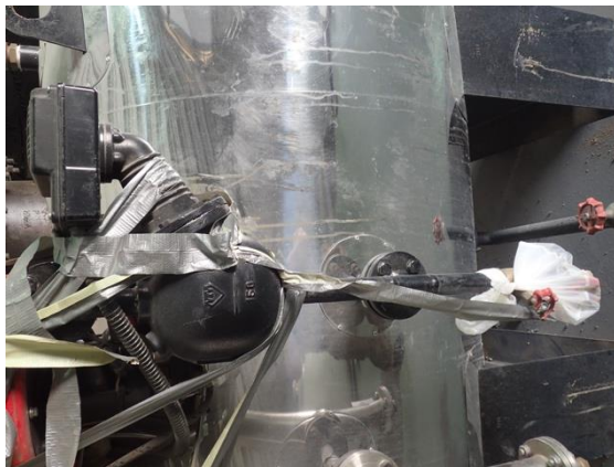
Figure D.36.28 Series 150SJ Low Water Cut-Off/Pump Generator
